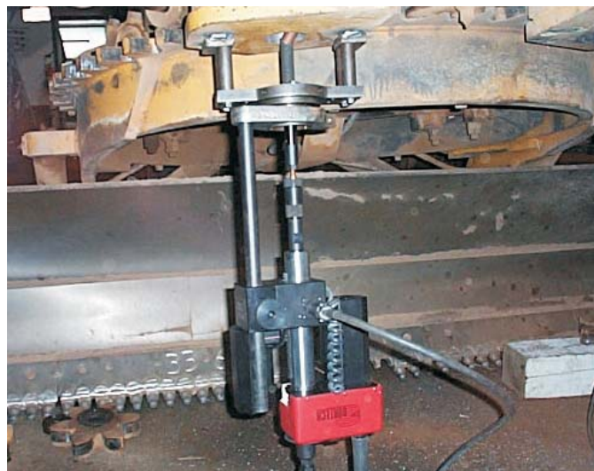
Repair on Earth Moving Equipment using Boretech Welder and Climax Boring Bar (BB2020)
